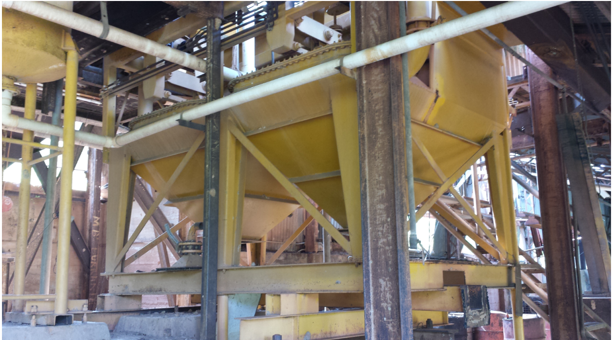
Figure 1 – Mt Wells processing plant
