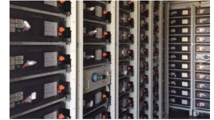
BATTERY ENERGY STORAGE SYSTEM (BESS) WA Western Power, $2m June 2016 – Mar 2017
