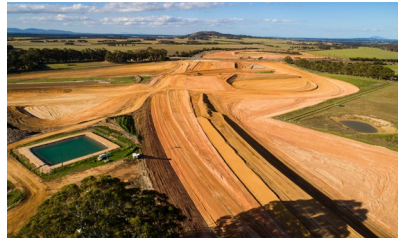
ALBANY RING ROAD PROJECT Albany, WA Main Roads WA, $55m Sep 2020 – Current
