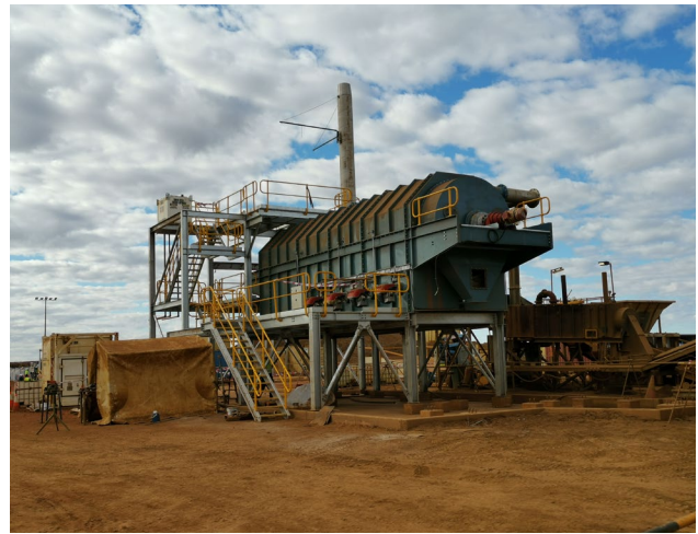
Concentrate Dryer in place
