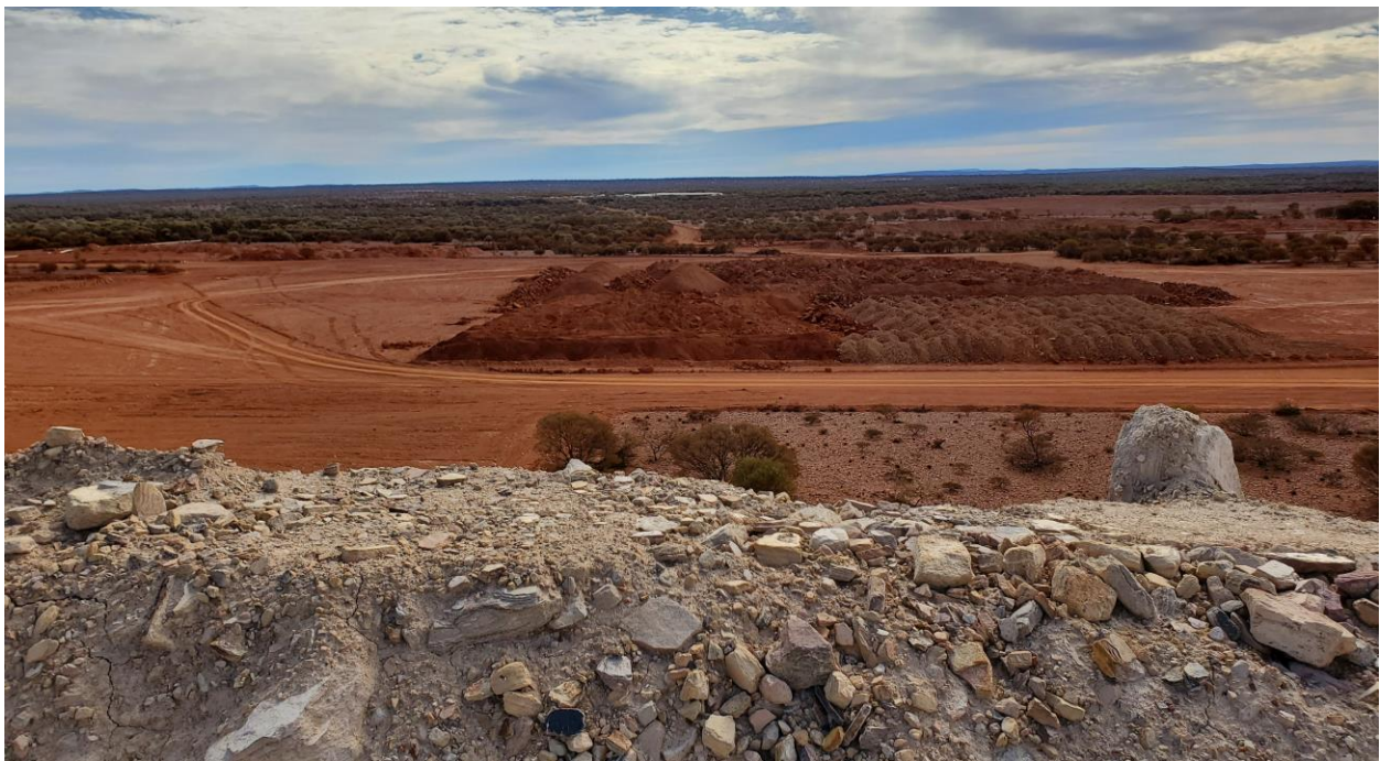
Figure 3. Cleared site of Abra's future processing plant (picture taken from the top of the ROM pad).
