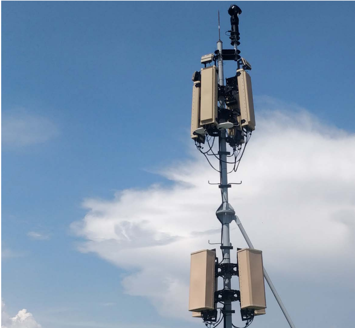
Image: DroneSentry™ deployed during the 2Q21 quarter
