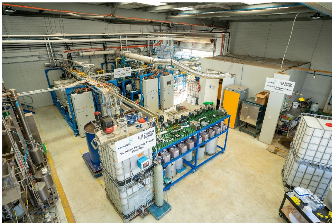
Figure 1 – Overview of Pilot Plant
