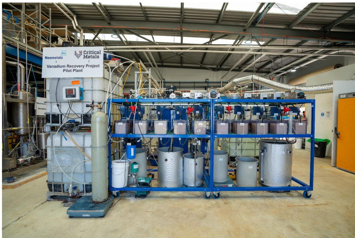
Figure 2 – Solvent Extraction section of Pilot Plant
