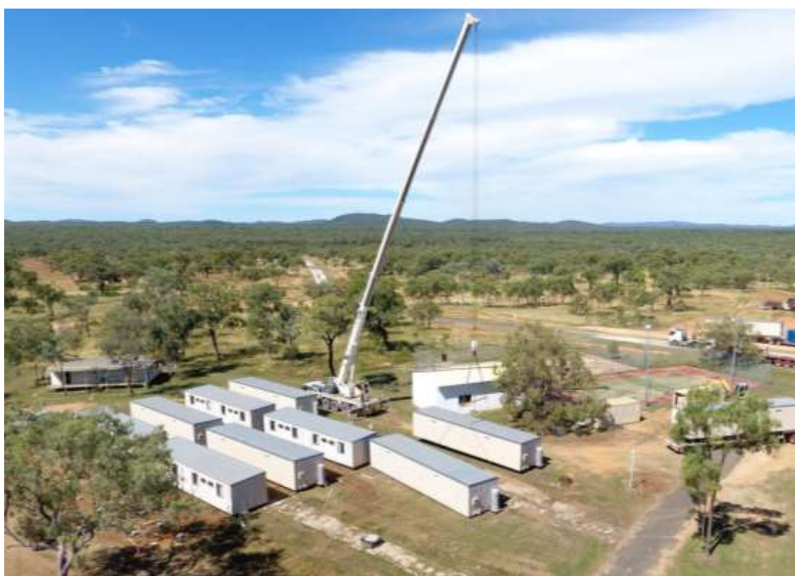
Figure 1: Expansion of accommodation camp at Oaks Rush, Kidston
