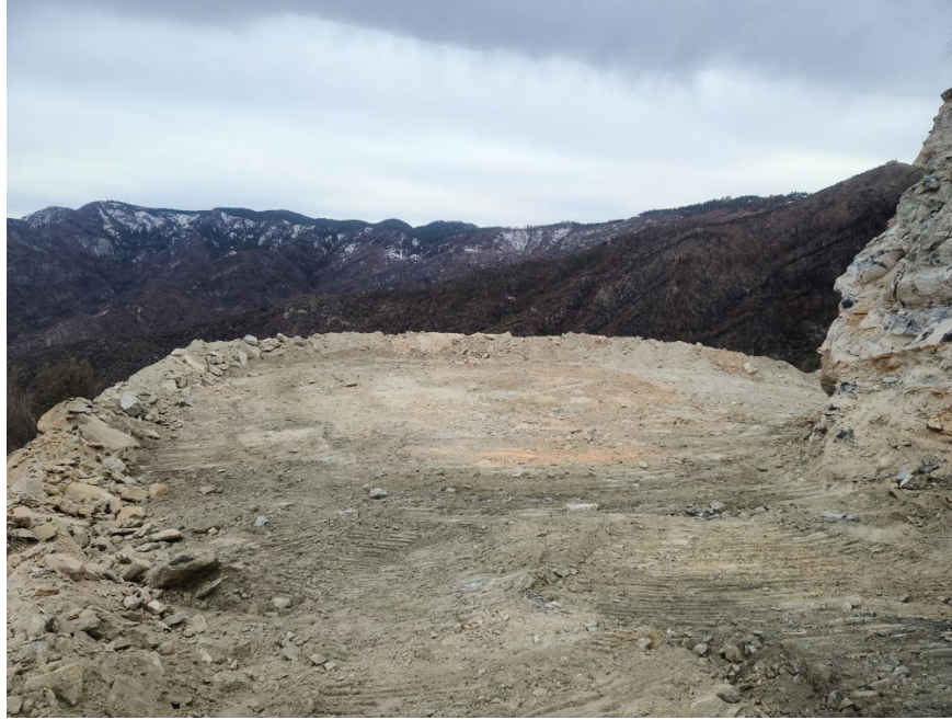
Figure 2 - Completed new pad in South Zone ready for the additional drilling rig
