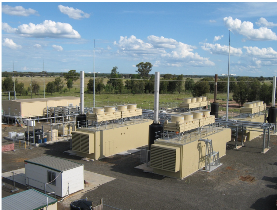
Wilga Park Power Station
