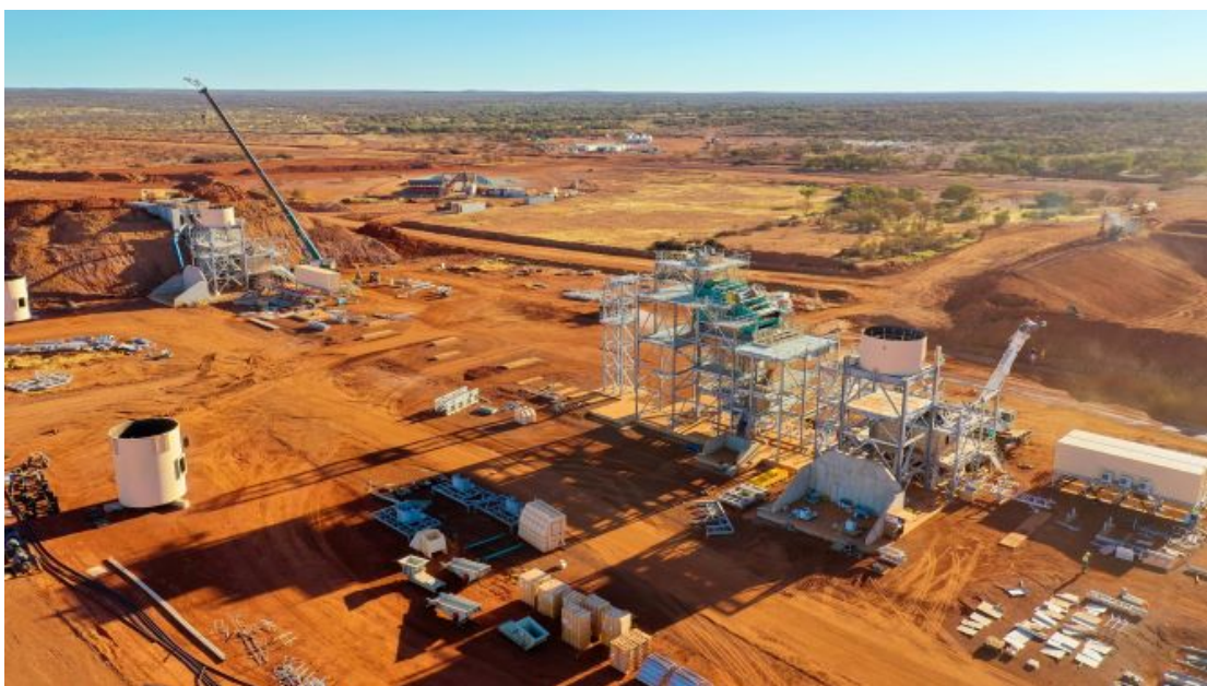
Primary, secondary and tertiary crusher installation
