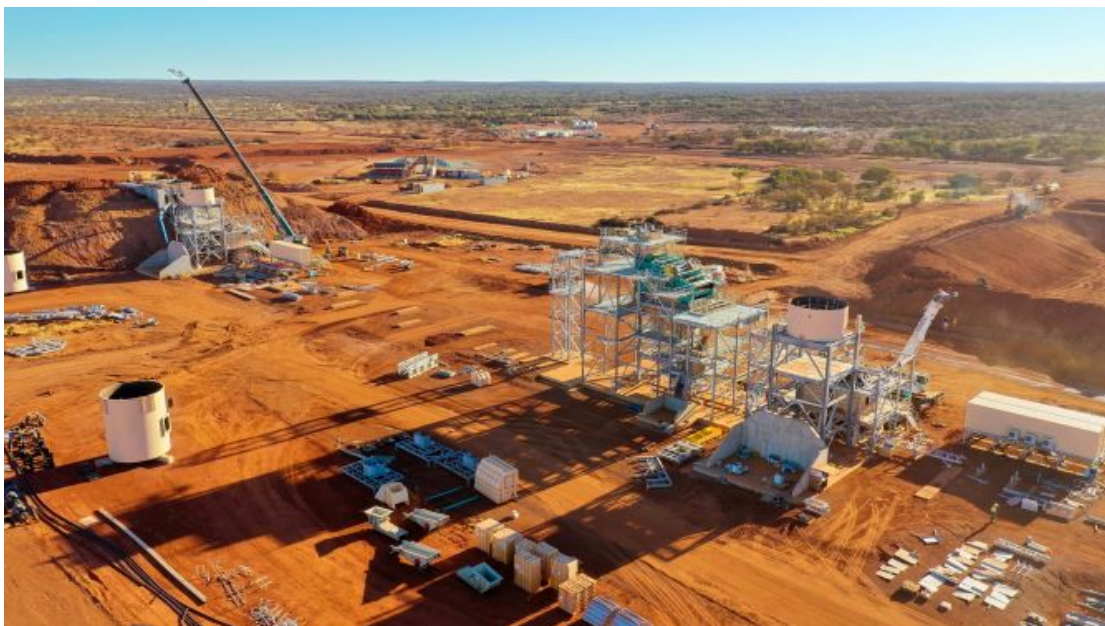
Primary, secondary and tertiary crusher installation
