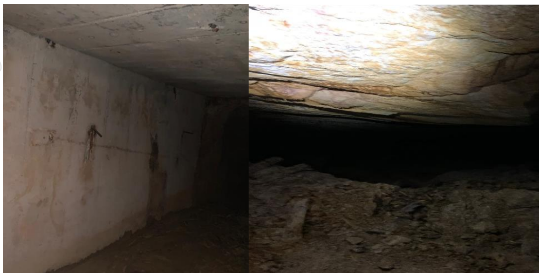
Image 4: Good condition reported of the Qala Adit shaft infrastructure (left) and the K9A hanging wall
