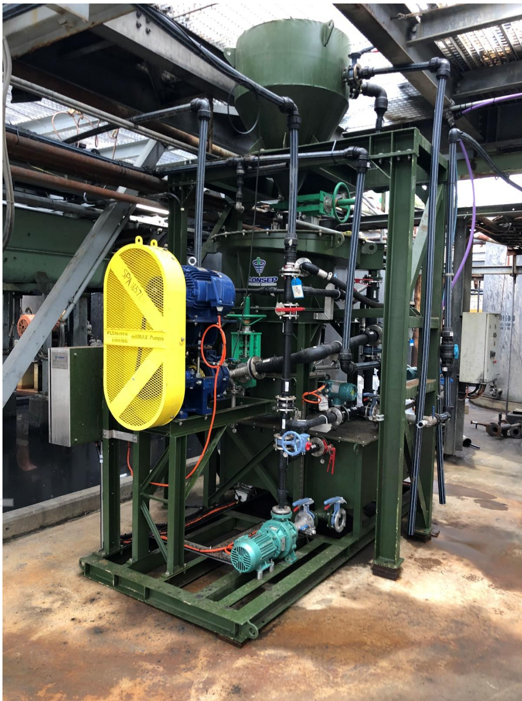
Figure 3 Consep Acacia Reactor installed at Hillgrove
