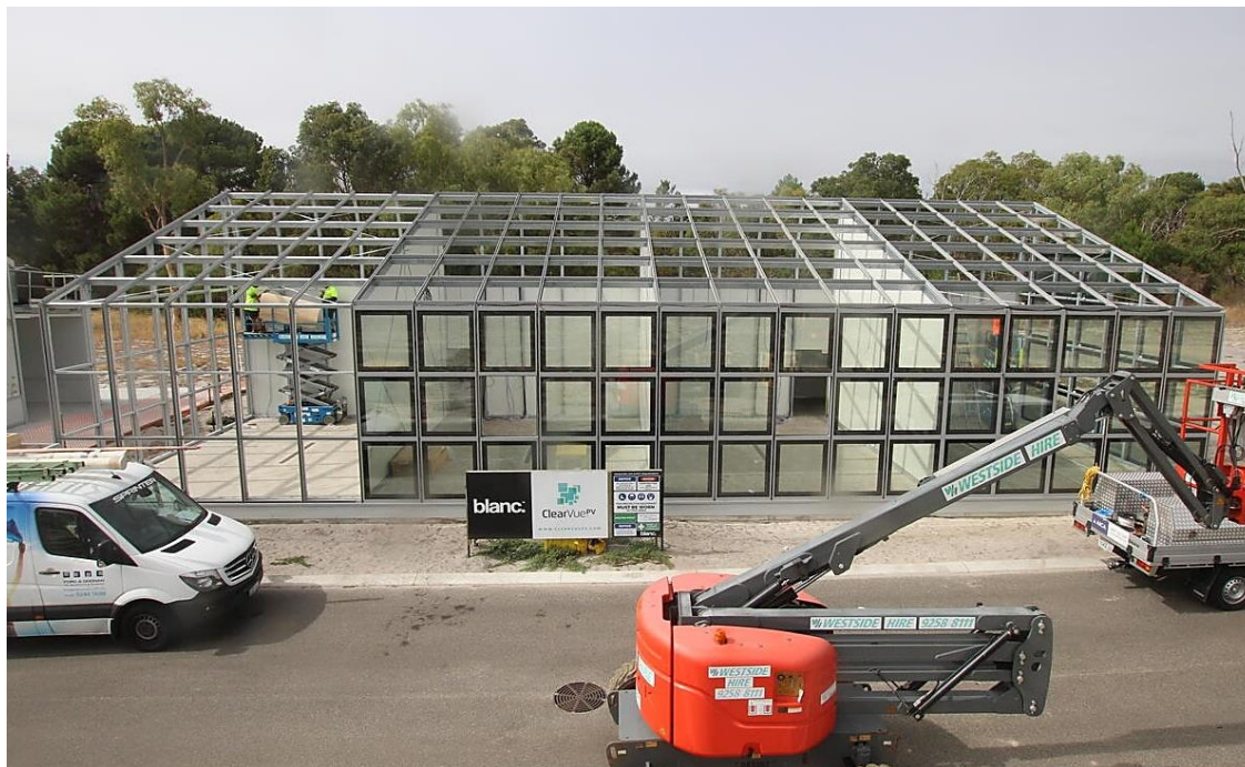
ClearVue's PV glazing being installed onto ClearVue's solar greenhouse at Murdoch University, Western Australia.
