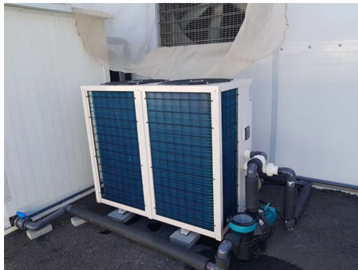
Figure 1: Heat pump and water tank (on the left) chamber installed at My Green Fields cannabis farm to be used for temperature control
