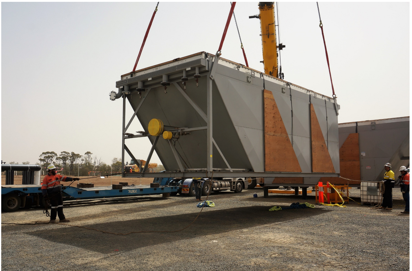
Procurement of long-lead items is underway for the expansion of Roma North to 24 TJ/day. This includes compressor modules such as the one pictured, which was delivered during construction of the existing facility.
