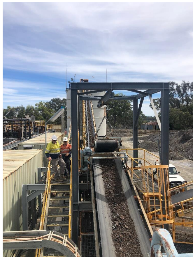
Figure 4 Crushed ore being fed into ore bin
