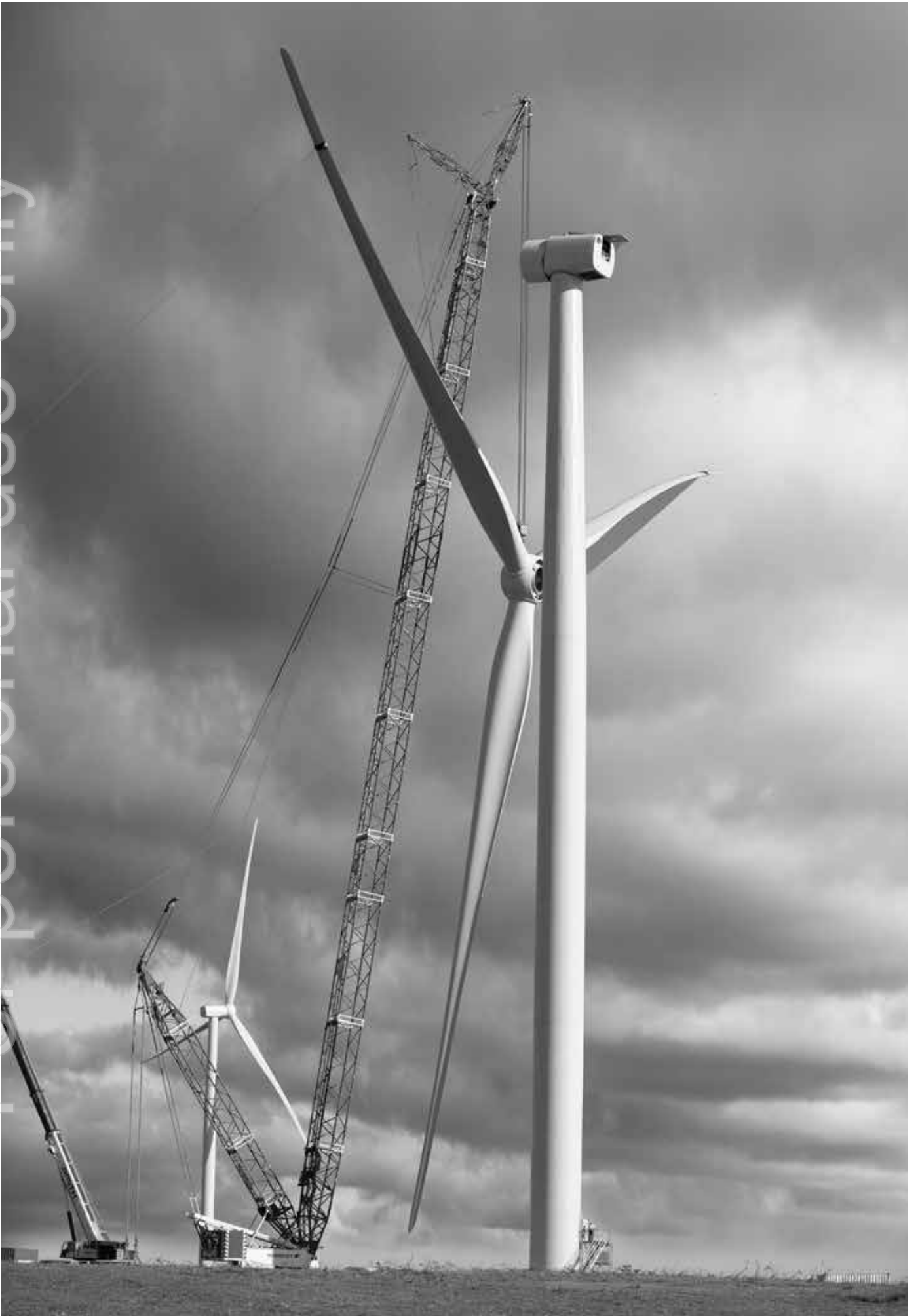
Erecting one of Waipipi Wind Farm's 31 turbines 7 kilometres southeast of Patea. The blade tip reaches 160 metres from the ground
