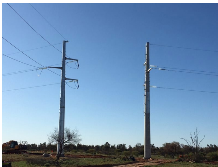
Figure 11: New transmission line
