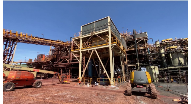
Figure 13: Jameson Cell steelwork
