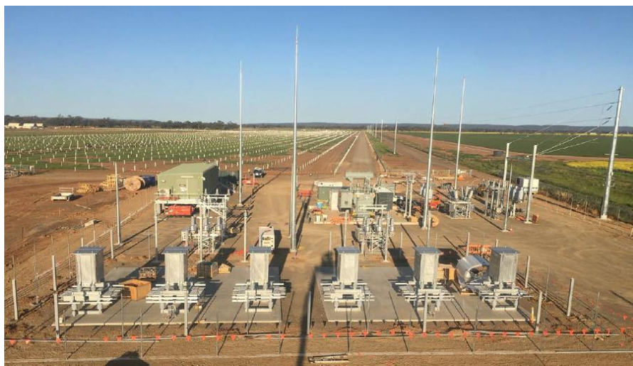
Figure 1. Jemalong Solar Project Substation Site
