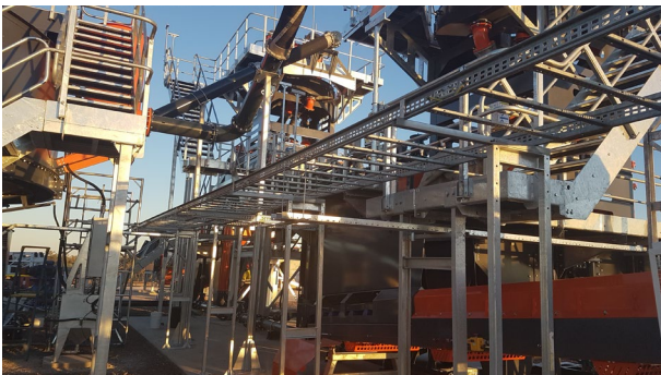
Figure 1 – View from within completed Start-up Plant at Ardmore
