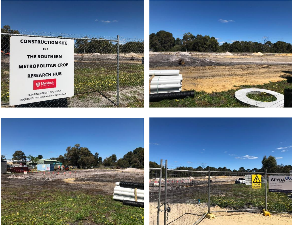
Site preparations at Murdoch University for new greenhouses, including the ClearVue CRC-P supported greenhouse.
