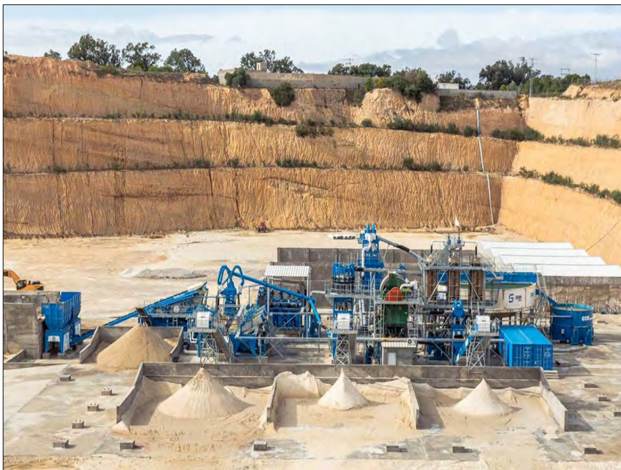
Figure 3.42 Silica sand plant
